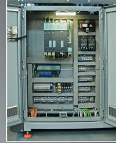
* Elektrik Panosu Electrical Cabinet
